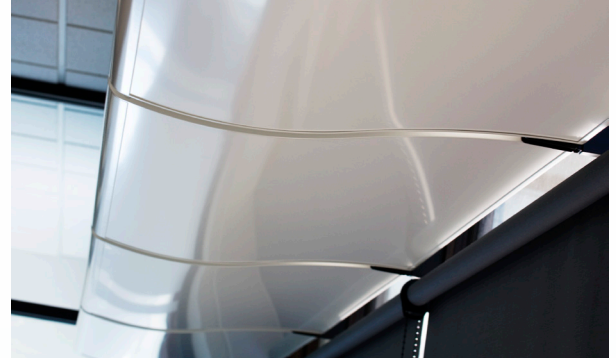
Continuous run installation
